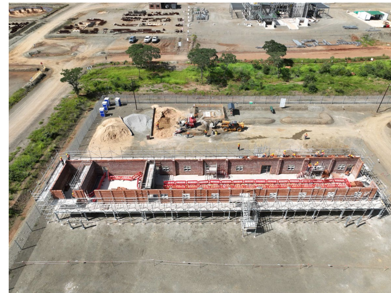
MV Substation Building
