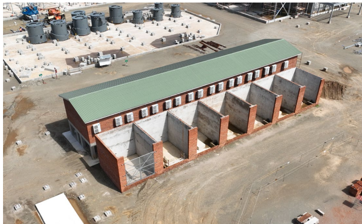
Wet End LV Substation
